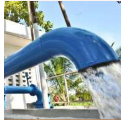
Water Supply Network through Automatic Pumps. Sewerage Disposal System.
